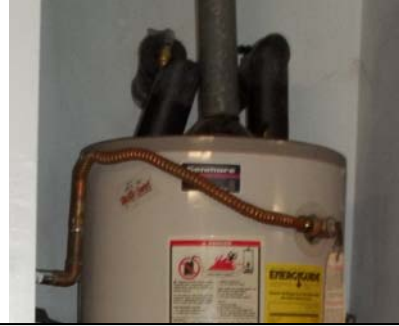
T&P drain line on water heater runs uphill inhibiting function.
