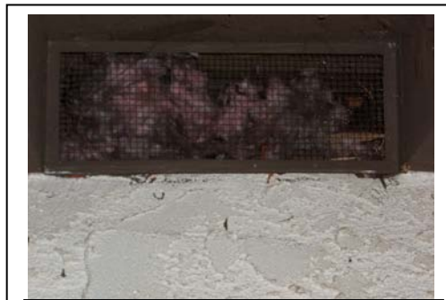
Insulation is blocking attic vents.
