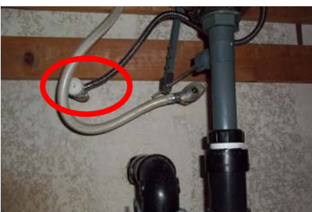
Corrugated angle stops have a tendency to leak or burst.
