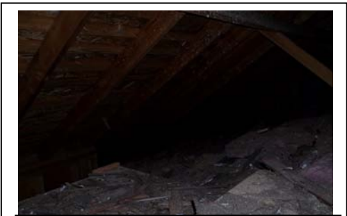
Debris is present in the attic from roof replacement.
