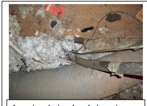
Low insulation levels in attic.
