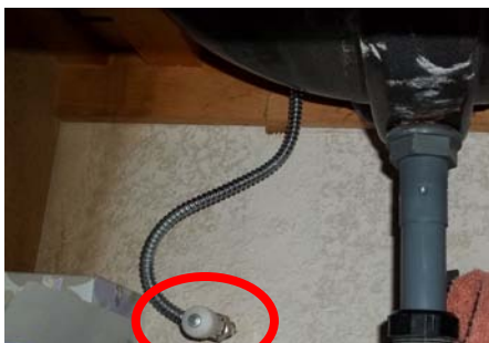
Corrugated angle stops have a tendency to leak or burst.
