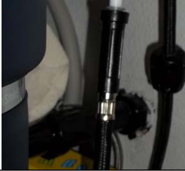
Sheet rock penetrations represent air loss. Sealing is required.
