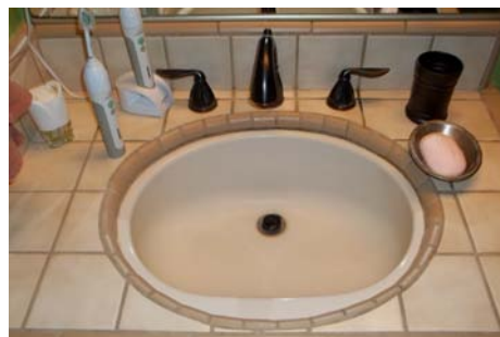
Overflow drain on this style sink has a tendency to rust through.
