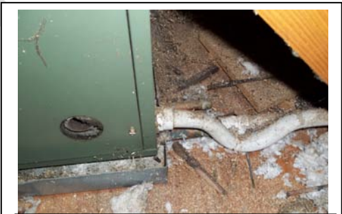
Debris is present in the condensate drain pan.
