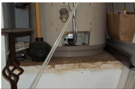
The water heater is missing a drain pan as required by code.
